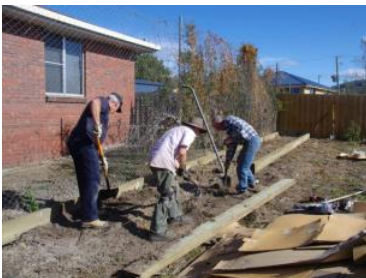
Above: Willing workers preparing the ground just prior to installation of the treated sleepers
